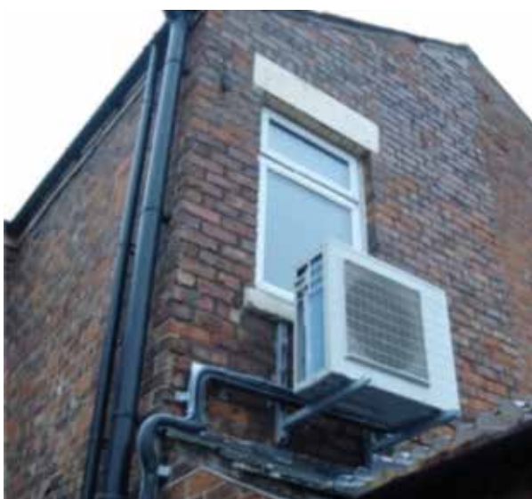
Figure 32: Picture of the installed hybrid heat pump module.
