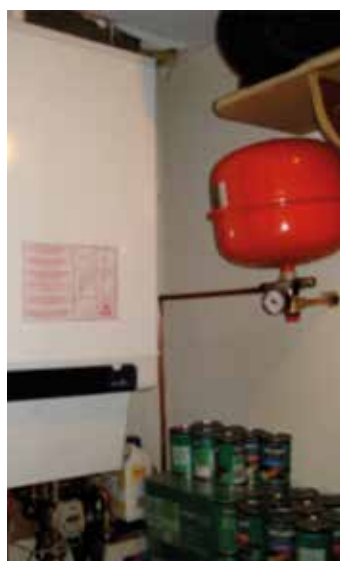
Figure 33: Picture of the indoor hybrid gas boiler and heat pump module (field test setup).
